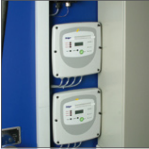
Gaswarnanlage Gas detection and alarm system
