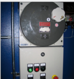
Ex Steuerung Flameproofed installations and controls
